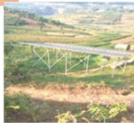
Required solar panel to power the pump
